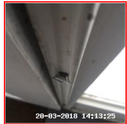
1.1.2 Damaged By Yale Lock Security Bar Not Fully Secured
