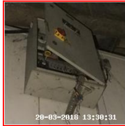
7.13.1 Side Electrical Box - Loose Wires And Cobwebs
