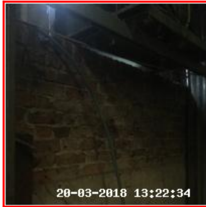
7.5.1 Pointing Chipped, Bricks Chipped
