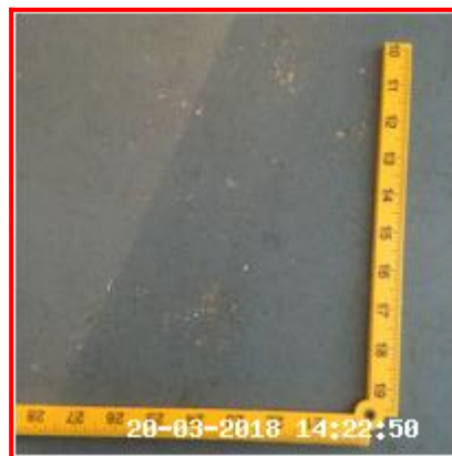
1.7.1 Indentations RHS Of Kitchen And By Warehouse Door Worn Patches To All Areas
