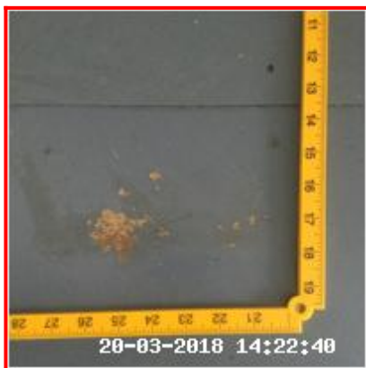
1.7.1 Indentations RHS Of Kitchen And By Warehouse Door Worn Patches To All Areas
