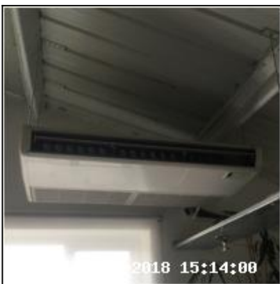
6.12 Air Conditioning Unit
