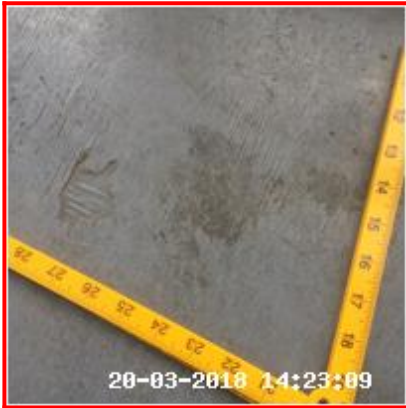
1.7.1 Indentations RHS Of Kitchen And By Warehouse Door Worn Patches To All Areas
