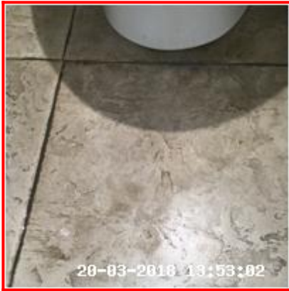
5.5.1 Wet In Front Of Toilet
