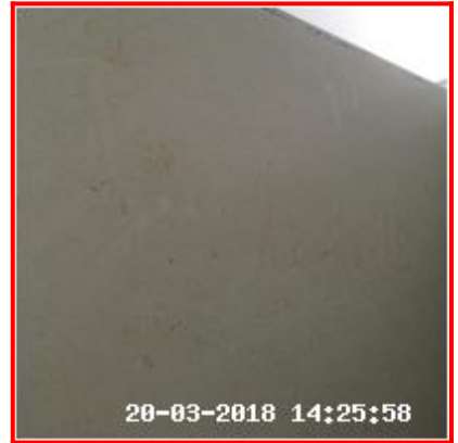
1.9.1 Rust Spots To Face
