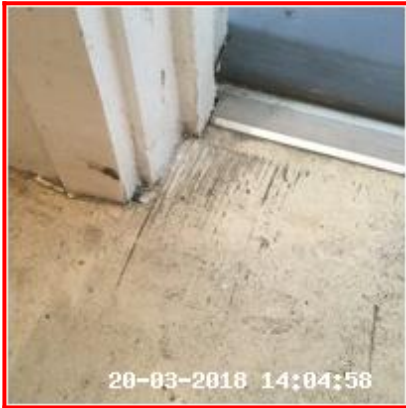
4.5.1 Scratched By Door And Toilet
