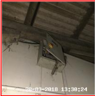
7.13.1 Side Electrical Box - Loose Wires And Cobwebs
