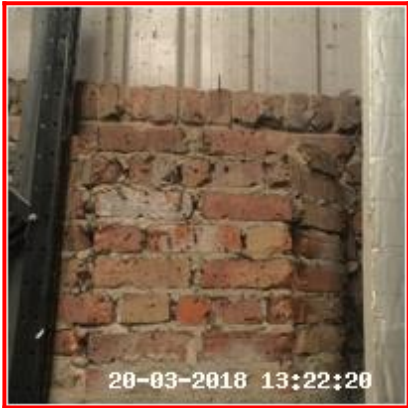
7.5.1 Pointing Chipped, Bricks Chipped
