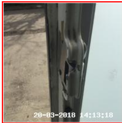
1.1.2 Damaged By Yale Lock Security Bar Not Fully Secured
