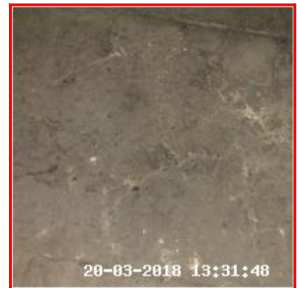
7.10.1 Cracked And Chipped LHS Of Large Fridge Unit
