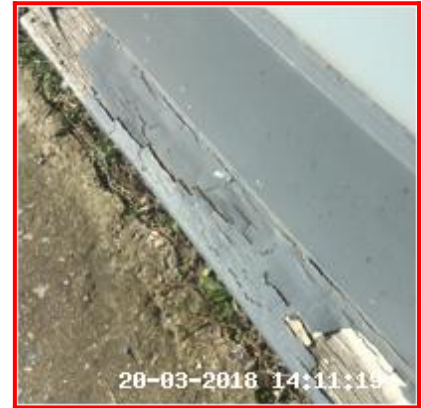
1.1.2 Heavily Weathered To Exterior
