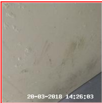
1.9.1 Rust Spots To Face
