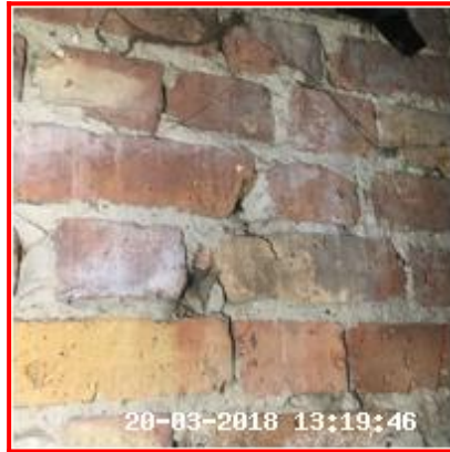
7.5.2 Brick Areas - Pointing Chipped, Bricks Chipped
