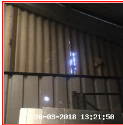
7.5.1 Holes To RHS Cladding
