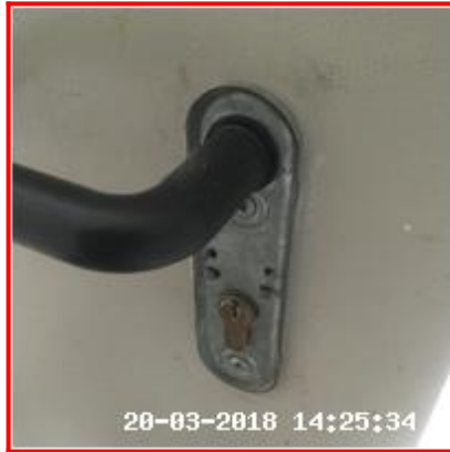
1.9.1 Lower Rear Worn Rear Handle Facia Missing
