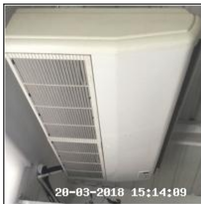
6.12 Air Conditioning Unit
