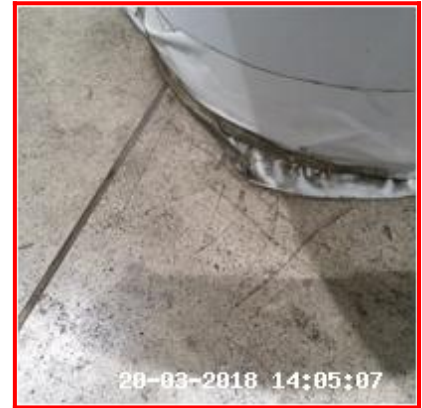
4.5.1 Scratched By Door And Toilet
