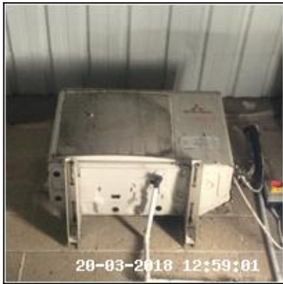
7.11 Air Conditioning Unit - Front
