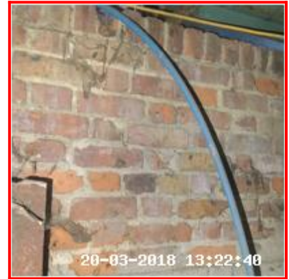
7.5.1 Pointing Chipped, Bricks Chipped
