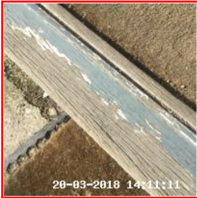
1.1.2 Heavily Weathered To Exterior
