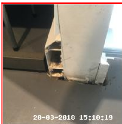
6.3.1 Both Ends By Stairs Missing
