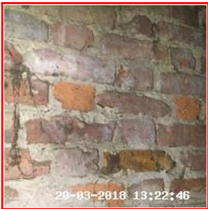
7.5.1 Pointing Chipped, Bricks Chipped
