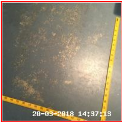
2.6.1 Heavily Worn To Centre
