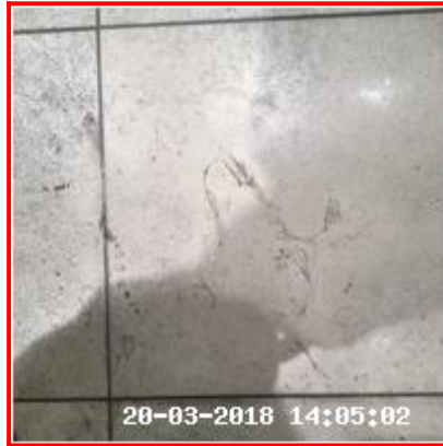
4.5.1 Scratched By Door And Toilet
