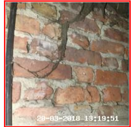
7.5.2 Brick Areas - Pointing Chipped, Bricks Chipped
