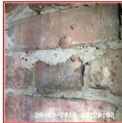
7.5.2 Brick Areas - Pointing Chipped, Bricks Chipped
