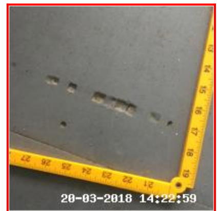
1.7.1 Indentations RHS Of Kitchen And By Warehouse Door Worn Patches To All Areas
