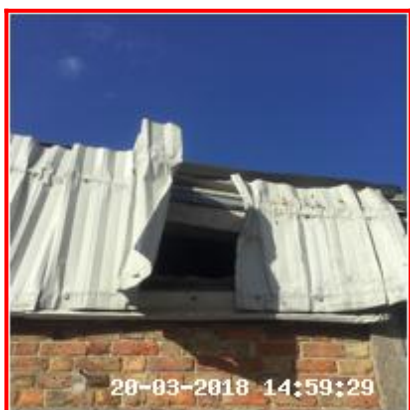
8.1.1 Cladding Damaged Above Disused Toilet
