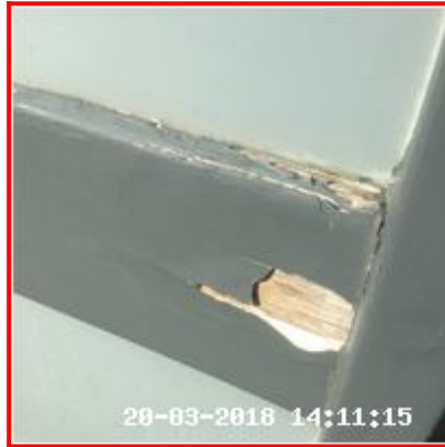
1.1.2 Heavily Weathered To Exterior
