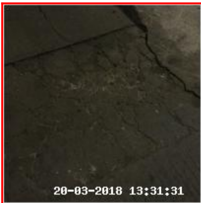
7.10.1 Cracked And Chipped LHS Of Large Fridge Unit
