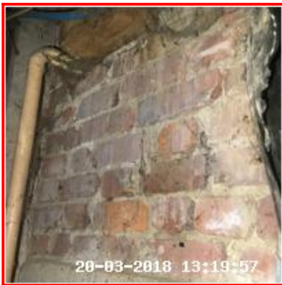
7.5.2 Brick Areas - Pointing Chipped, Bricks Chipped
