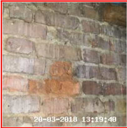
7.5.2 Brick Areas - Pointing Chipped, Bricks Chipped
