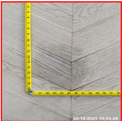
5.1.1 Stain By Balcony Door
