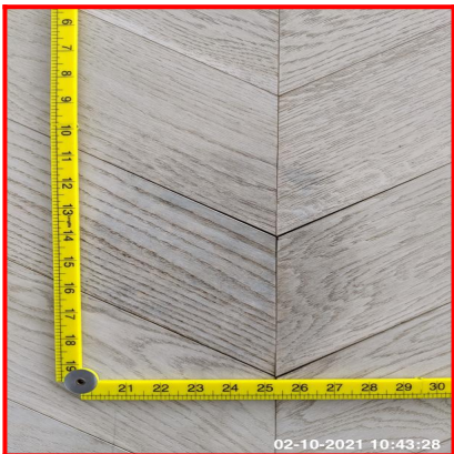
5.1.1 Stain By Balcony Door
