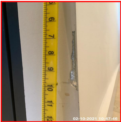
5.1.3 Large Chip LHS Of Fridge
