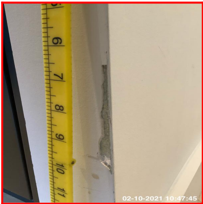
5.1.3 Large Chip LHS Of Fridge
