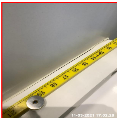
3.1.1 Sealant Damaged To Rear
