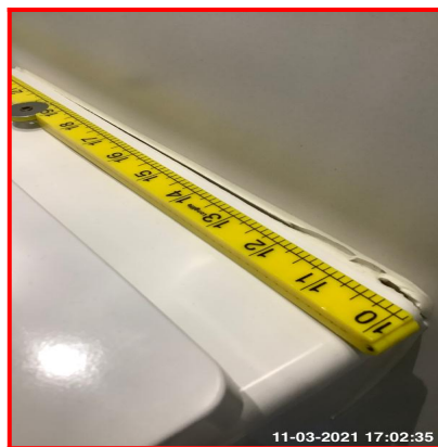
3.1.1 Sealant Damaged To Rear
