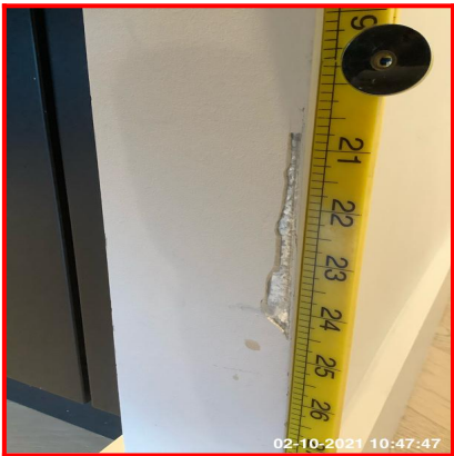
5.1.3 Large Chip LHS Of Fridge
